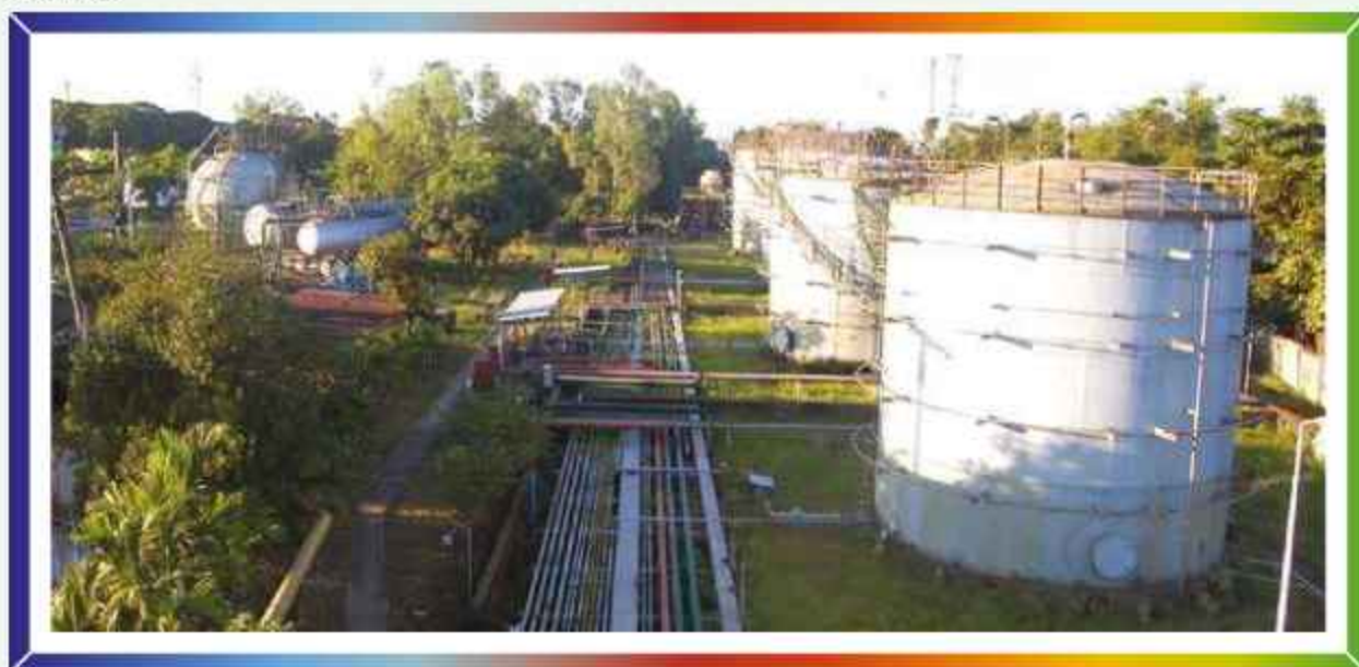
Kailashtila LPG Plant at Golappanj, Sylhet.
