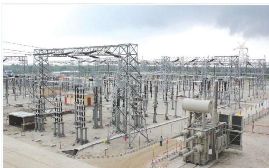
Figure 20: Bangladesh India Power Transmission Plant, Bheramara (Kustia)
