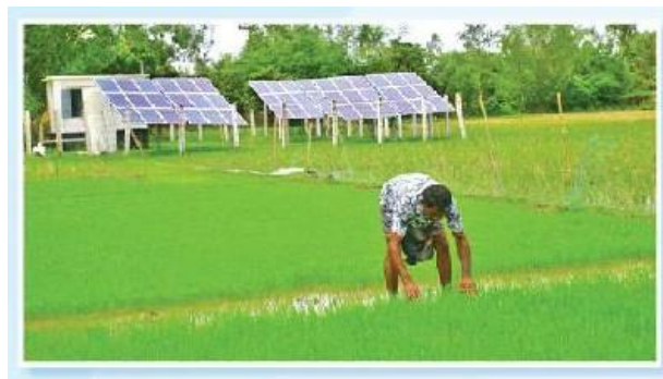
Figure 24: Solar Pump System in Rangpur District
